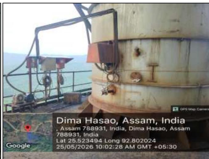
Coal mill stack monitoring platform
