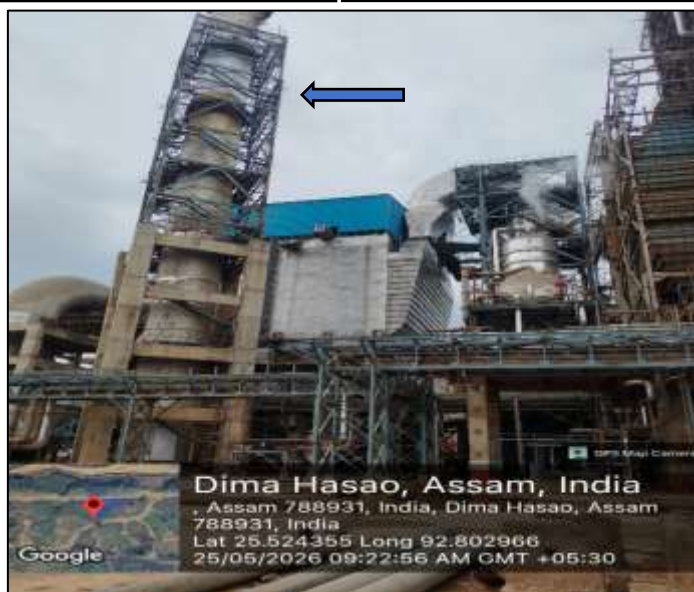
OCEMS at Cooler stack monitoring platform
