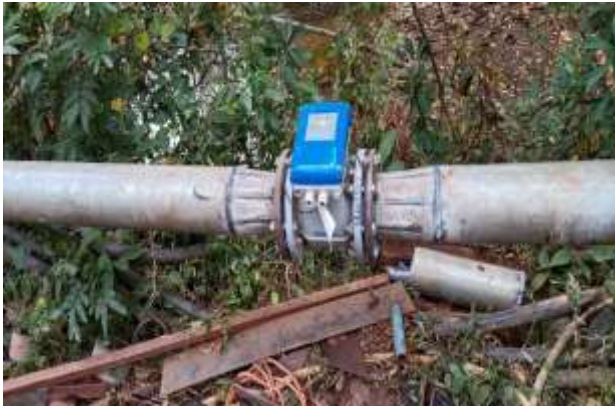
At Amrang Nala pump (Water Source)
