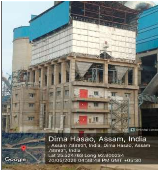
Photo Showing Raw Mill + Kiln RABH
