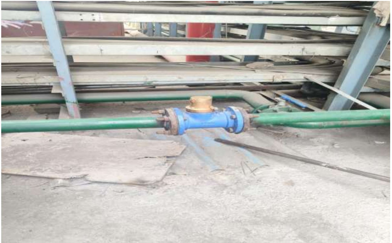
Preheater (Process Water)
