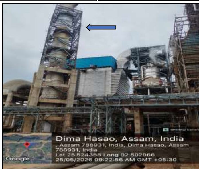
Cooler stack monitoring platform
