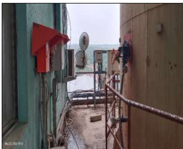
OCEMS at Raw mill+Kiln stack
