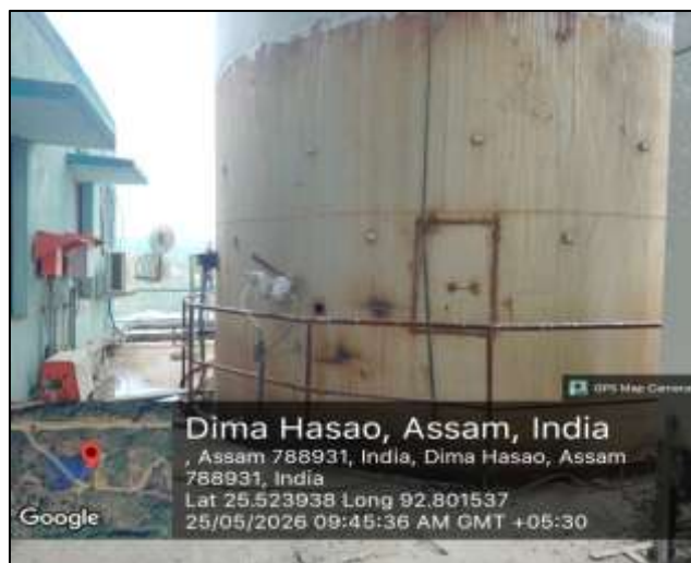
Raw mill+Kiln stack monitoring platform
