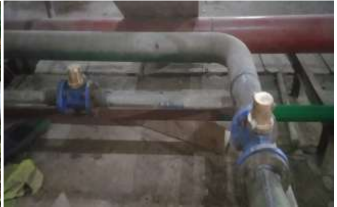
At ACC Pump house Process & Drinking Water
