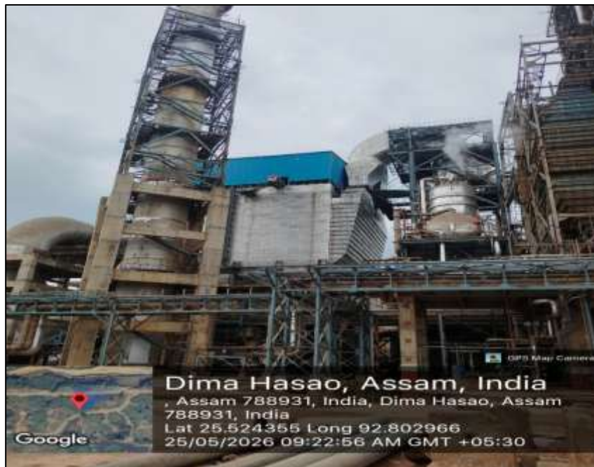
Photo Showing cooler ESP
